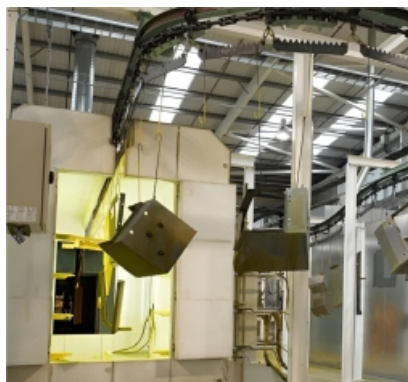
Automated Powder Coating
