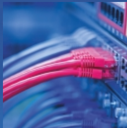
Data Transmission Cables
